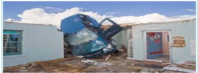
Figure 5: Damage caused by Tornadoes.
